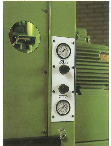
Control panel for table and infeed pressure bar adjustment.
