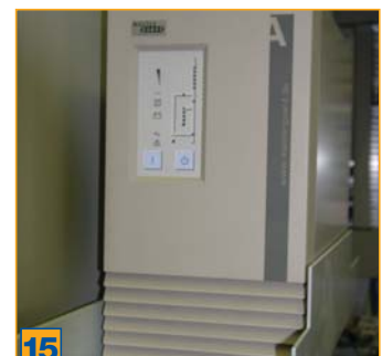
15 Uninterruptible power system (UPS) to eliminate faults in the event of mains power fluctuations and data loss following power failures
