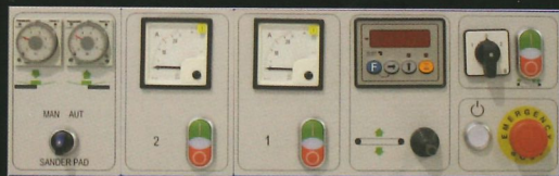
| S : CONTROL PANEL
