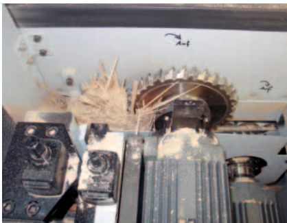
Broken splinters block the extraction hood - fire risk through friction of the rotating tool!
