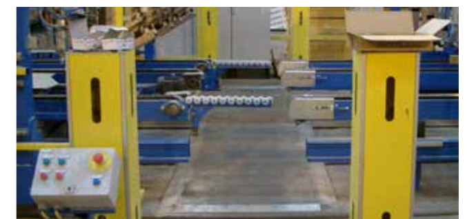
Light beams and safety mats between the stations.
