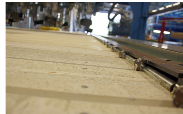
The cladding template makes the placing of timber exact and the nail pushers push the nails to exact depth unlike when nailing with traditional nailing guns.
