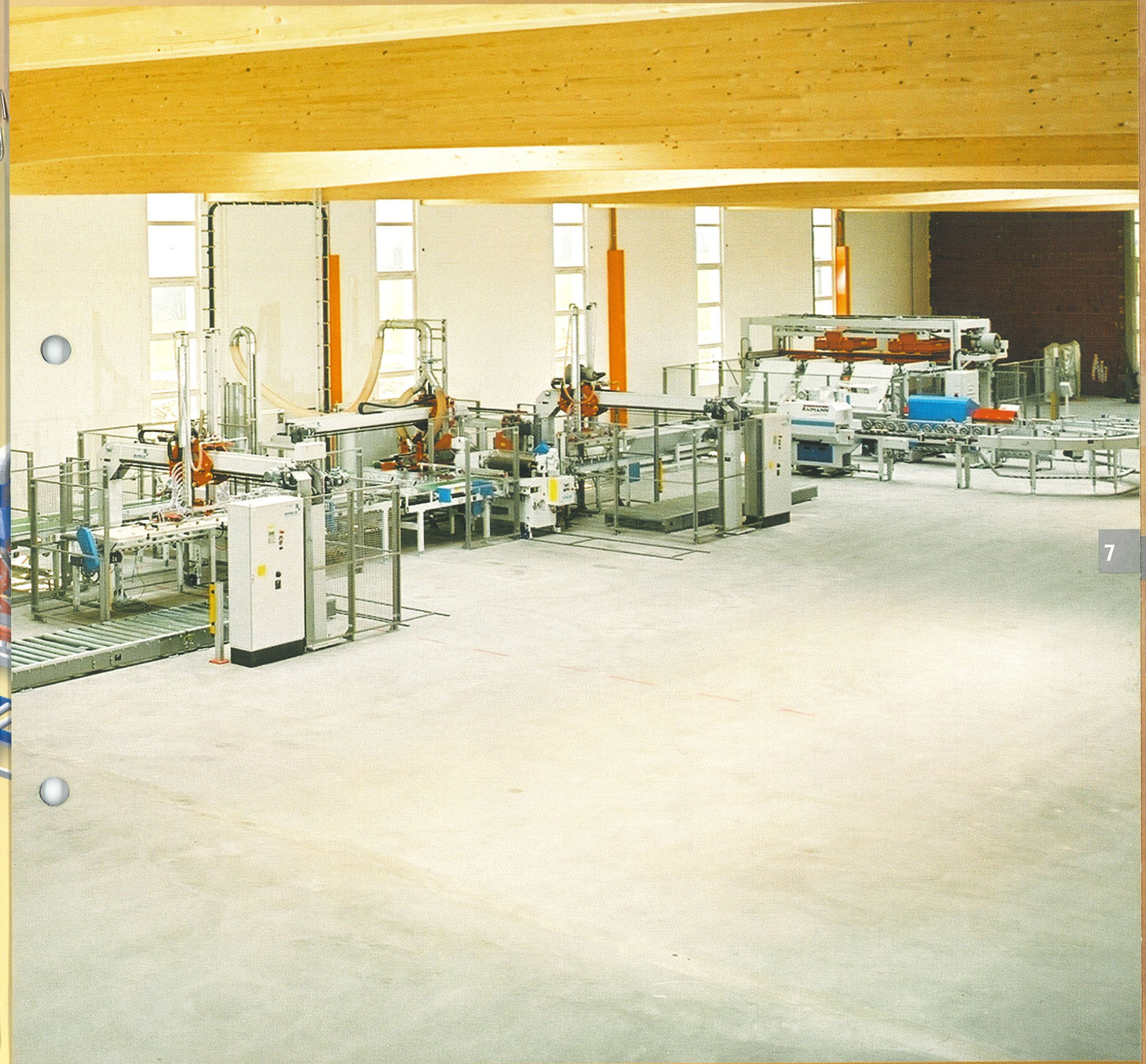
CORE LAYER PRODUCTION AND PRESS LINE
