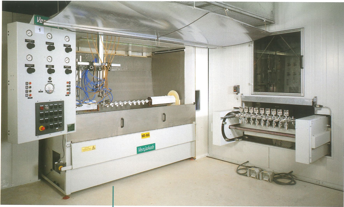
Automatic spindle machine (left) for coating hollow cylindrical components in combination with a vertical dryer
